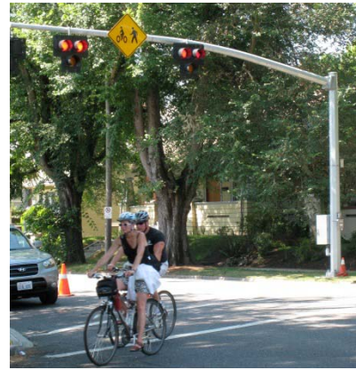
High Intensity Activated Crossing (HAWK) Beacon
