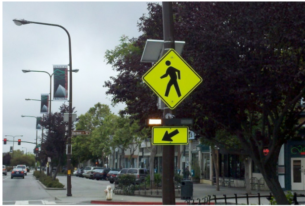
Rectangular Rapid Flashing Beacon
